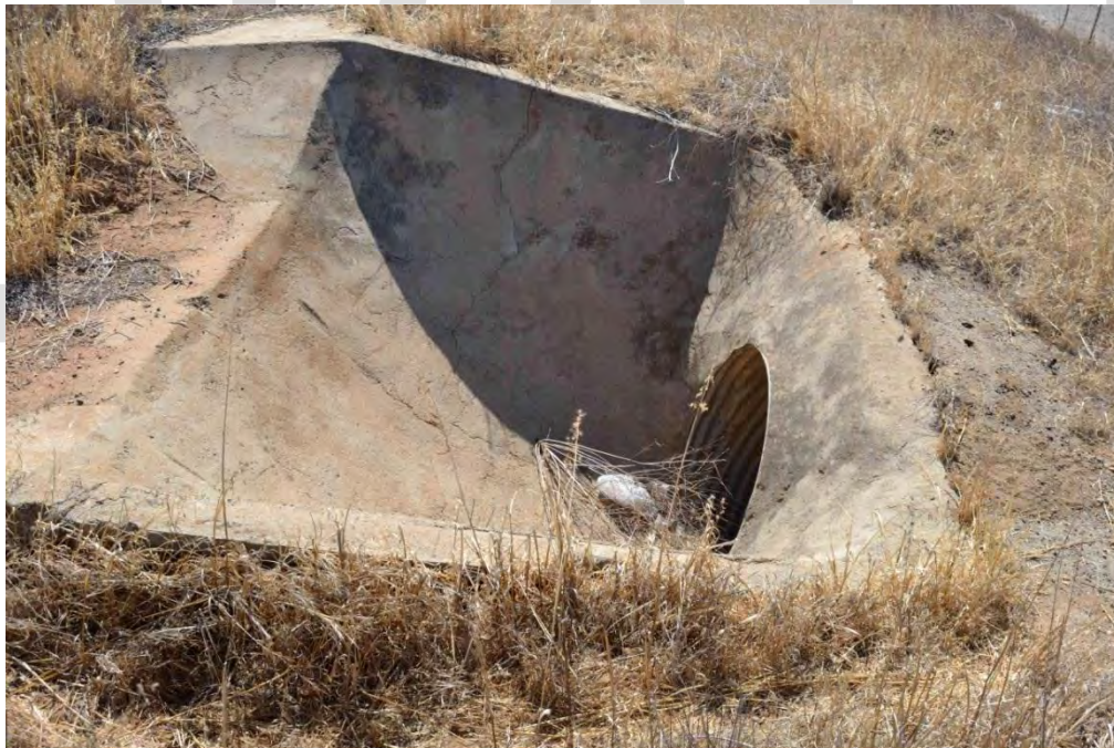
Figure 10. Looking south. This inlet is very steep and the sides are smooth concrete.
