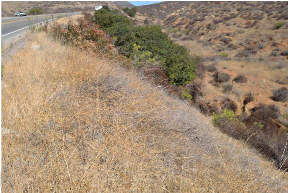
Figure 14. Looking northeast. The culvert outlet is at the bottom of the slope. The truck on opposite side of the road is above the opening to the culvert (figure 4) on the west side.
