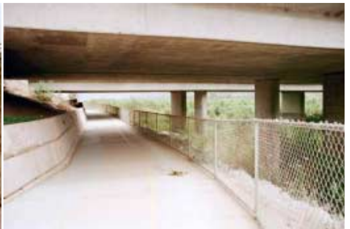
I-15 bridge over Lake Hodges/San Dieguito River, looking east from north side paved trail.
