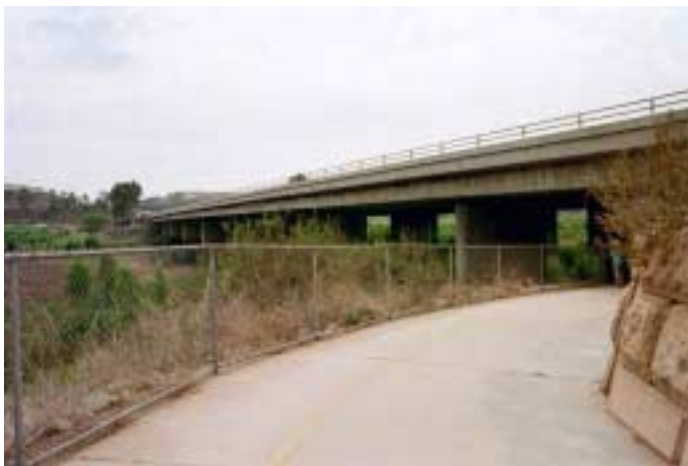
I-15 bridge over Lake Hodges/San Dieguito River, looking southwest from north side paved trail.
