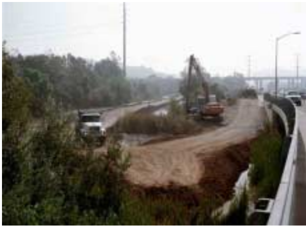
Dredging project in L-9 linkage, looking south from Sorrento Valley Rd bridge.
