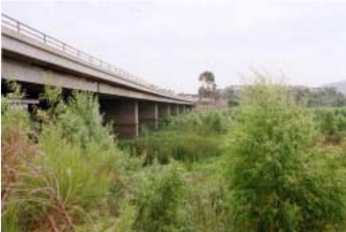
I-15 bridge over Lake Hodges/San Dieguito River, looking south from north side.
