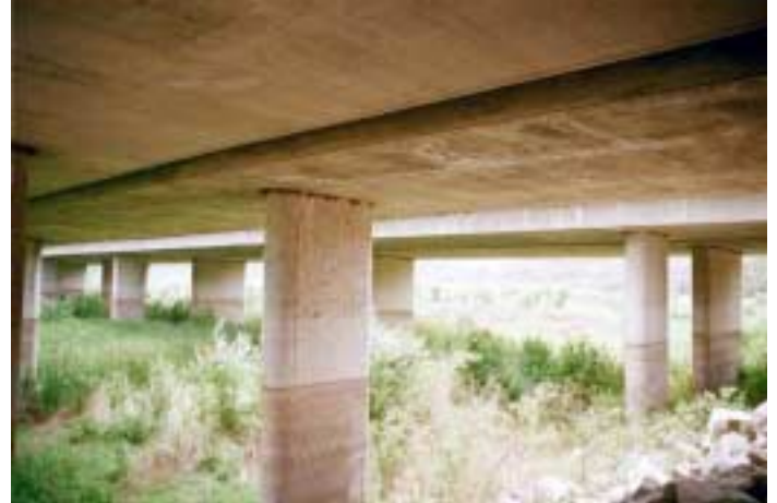
I-15 bridge over Lake Hodges/San Dieguito River, looking southwest from north side paved trail.
