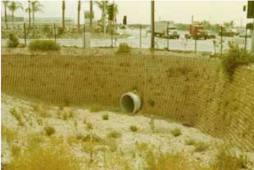
Culvert under Otay Mesa Rd. from the north side of the culvert, looking east.
